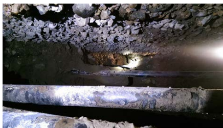
Figure 2. A large cavity formed under utility trench due to material escaping, Anzali Old quaywall.
