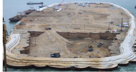
Figure 7. The final stages of building the island and the embankment within it.
