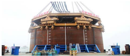
Figure 5. Guiding lines and vibration equipment for installing cylinders in the sea bed.
