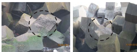
Figure 1. Breakage of Xbloc® armour units
