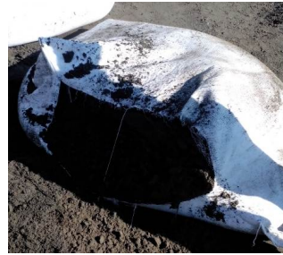
Figure 3. Tearing of bag due to weakness of geotextile
