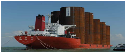
Figure 4. Carry the steel cylinders from the workshop to the construction site of the island.
