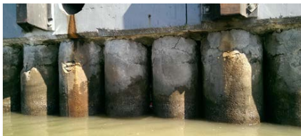
Figure 1. Open spaces between concrete piles, Anzali old quaywall.
