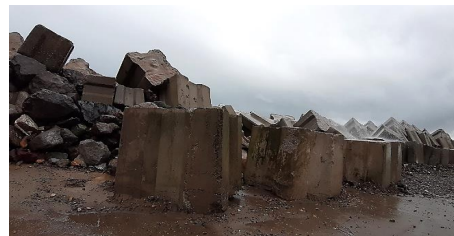
Figure 2. Sliding of antifer armour units (photo: January 2021, 21 st ).
