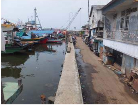
Figure 2. Pluit District is situated below sea level. The thin dyke protecting the settlement was raised by about a meter after the 2007 high tide event. The bay serves as a port for many fishing and work vessels (Photo: May 13, 2016).
