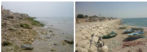
Figure 5. Erosion (left) and protection (right) at the downstream of Shioo port
