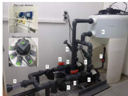
Figure 2. A view of the piping system, pot, sensors and data logger of the monitoring station
